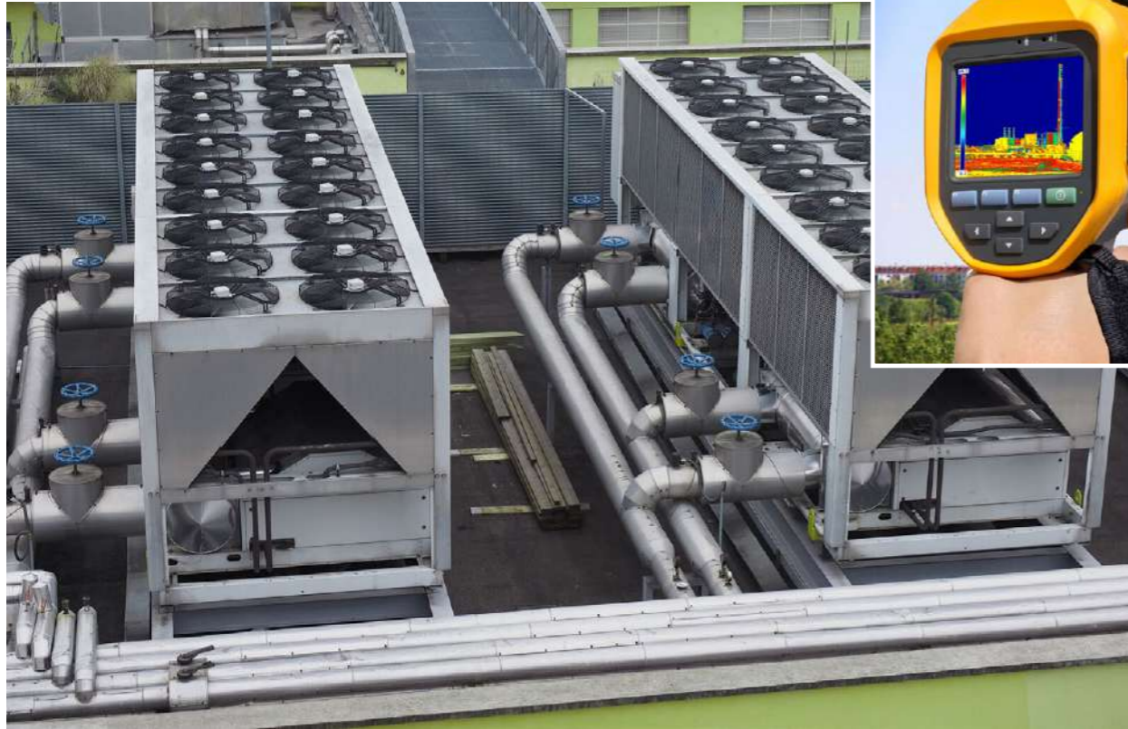
A heating ventilation and air conditioning device with fans on roof top
