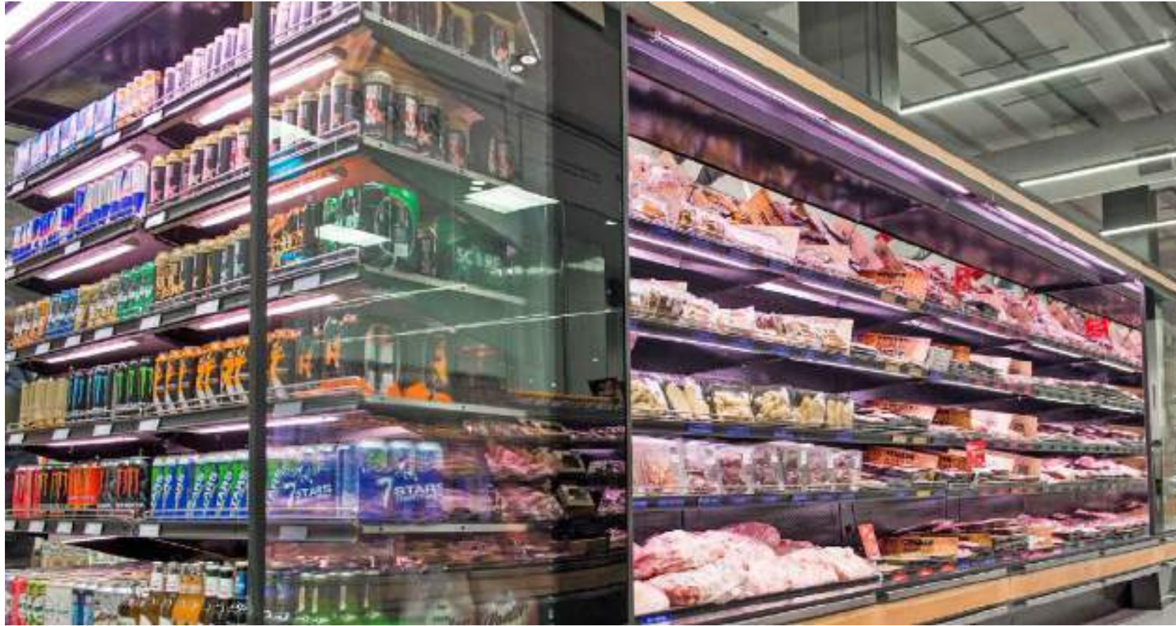
Shoprite Checkers with an Energy Partners refrigeration solution.
