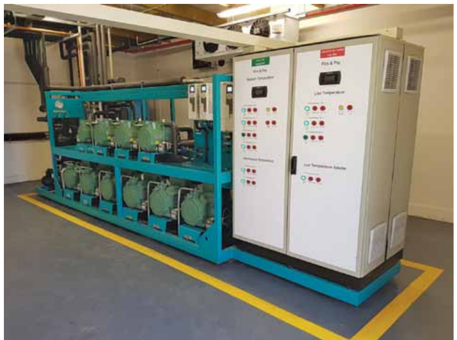
The CO 2 transcritical refrigeration pack was built by Sphere.
